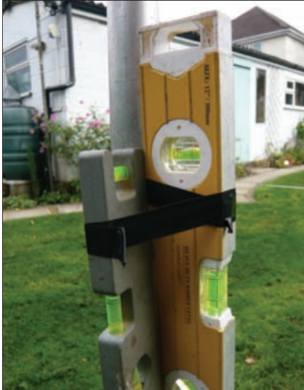
Two spirits levels to make sure the support pole is truly vertical when it's embedded in the ground.
